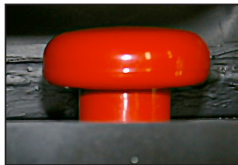
“Big Red Button” - Emergency Shut Off
